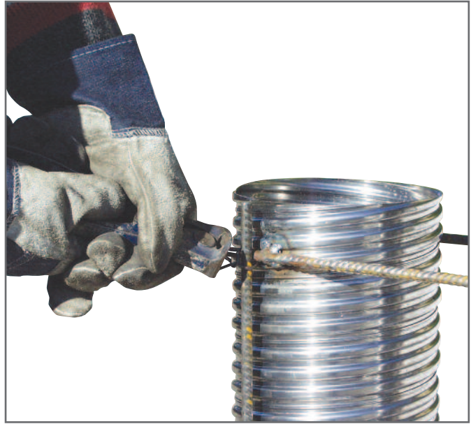
Fixing the anchoring set to the vertical pins of the frame after adjusting the correct height. This can be carried out before or after the setting of the top layer.
